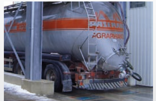
WWS installed flush floor, for dynamic weighing >>
