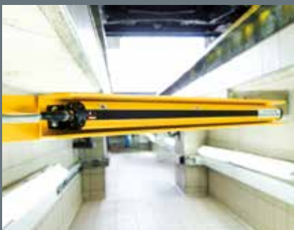
PSC1, pit safety protection, alongside
